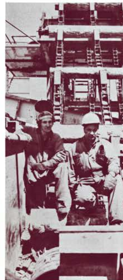
Welder Lyle Morrison and Millwright Del Virk, just finishing the installation of a shock absorber plate on the bumper of the log incline transfer of No. 4 Woodroom. As Del put it, "Just another lunch-hour job."
