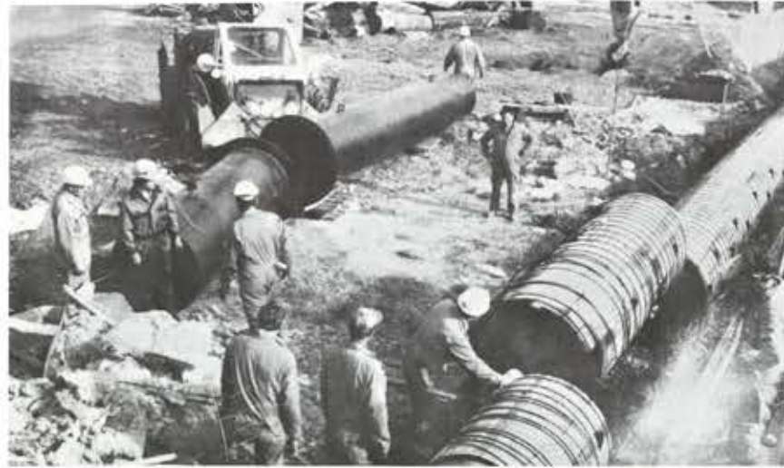
A nice way to spend Saturday morning! Carpenters and pipe-fitters from Maintenance replace a 30 foot section of Harmac's well water line.
